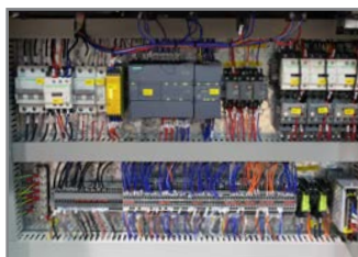
MACCHINA GESTITA DA PLC MACHINE CONTROLLED BY PLC
